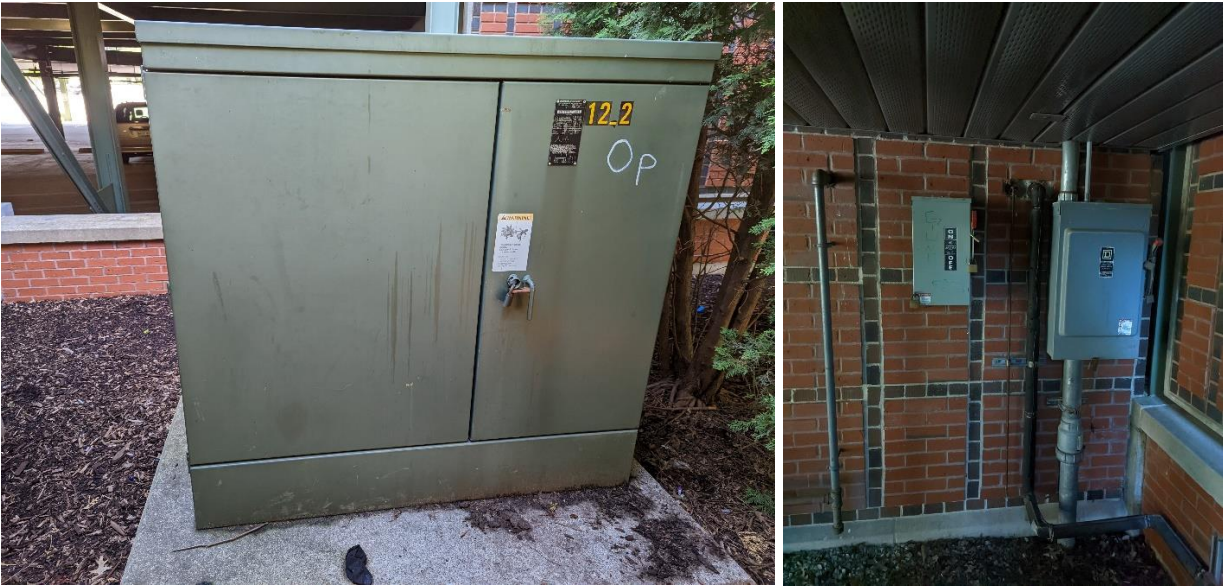
Figure 9 Oak St. Municipal Parking Lot Electrical Distribution Assets
